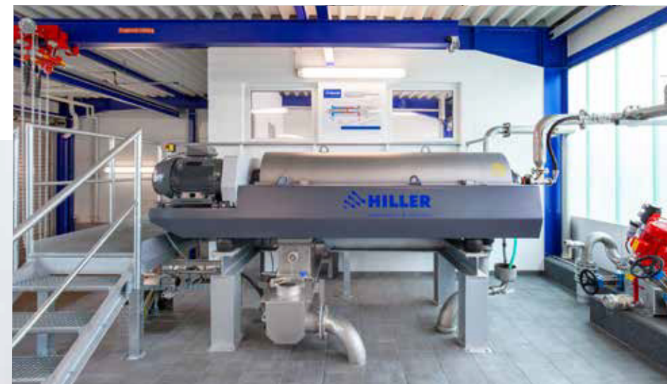
Hiller decanter in municipal wastewater treatment
